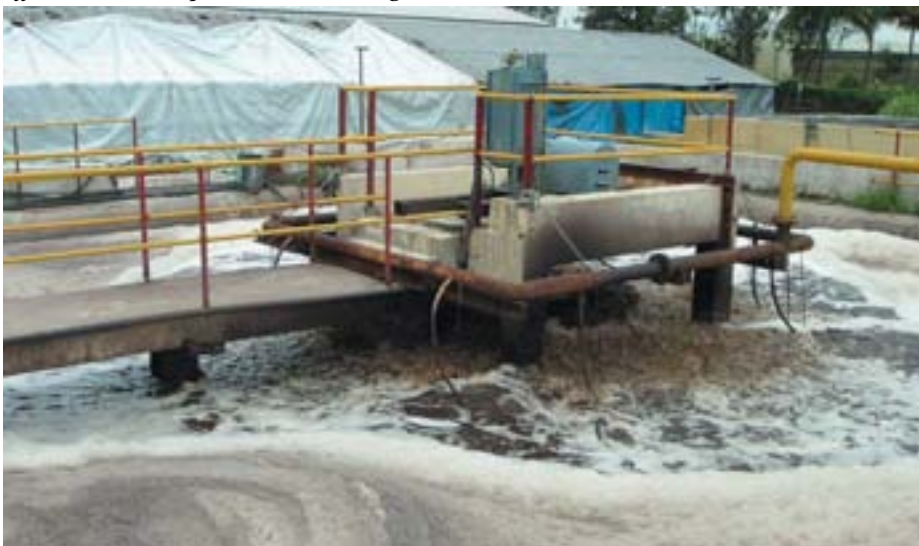
Effluent treatment plant at SSCL, Berigai.
